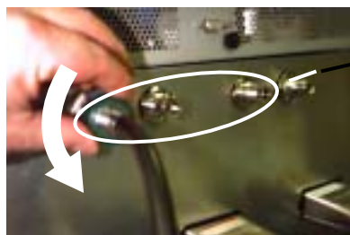
Pipeline Hoses Disconnected
